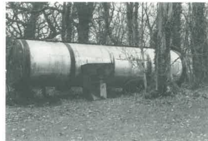
Water storage tank
